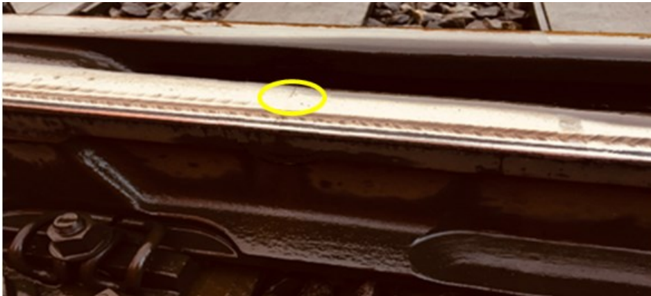
Transverse cracks on other running surfaces of the casting Defect code 722N
