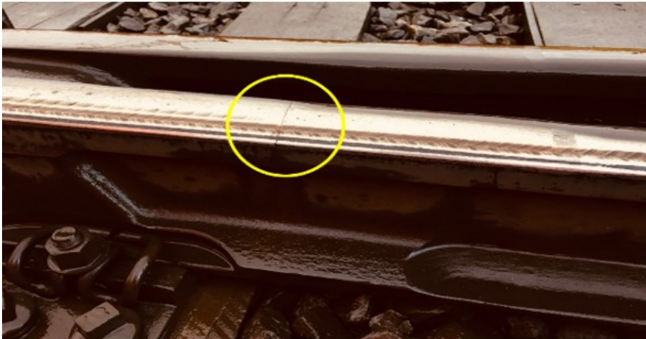
Transverse cracks on other running surfaces of the casting Defect code 732V
