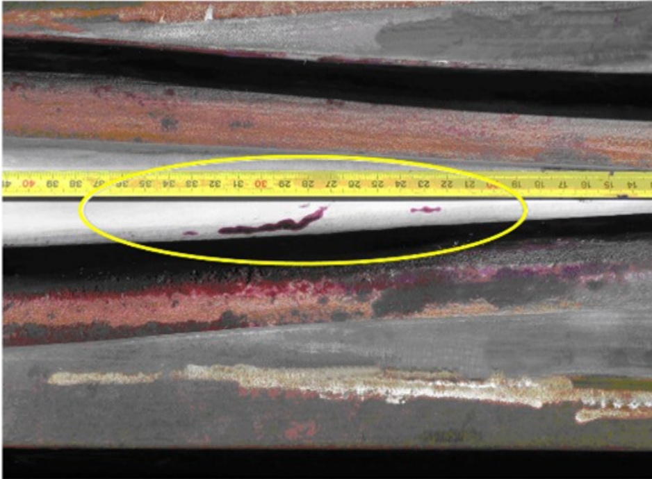
Longitudinal cracks on running surfaces in the crossing point-wing area Defect code 621N
