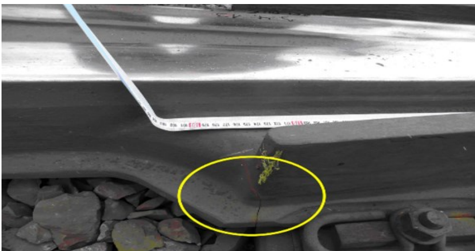
Transverse cracks on the casting Defect code 734V
